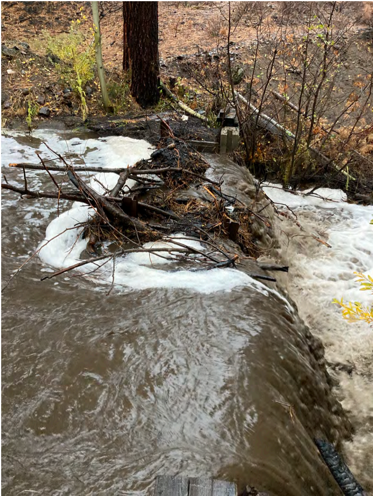
Photo 2: In October of 2021 a flash flood occurred in the Markleeville area including the Musser and Jarvis watershed. Debris from the flash flood covered the dam and intake structure, and sediment filled the intake pipe.
