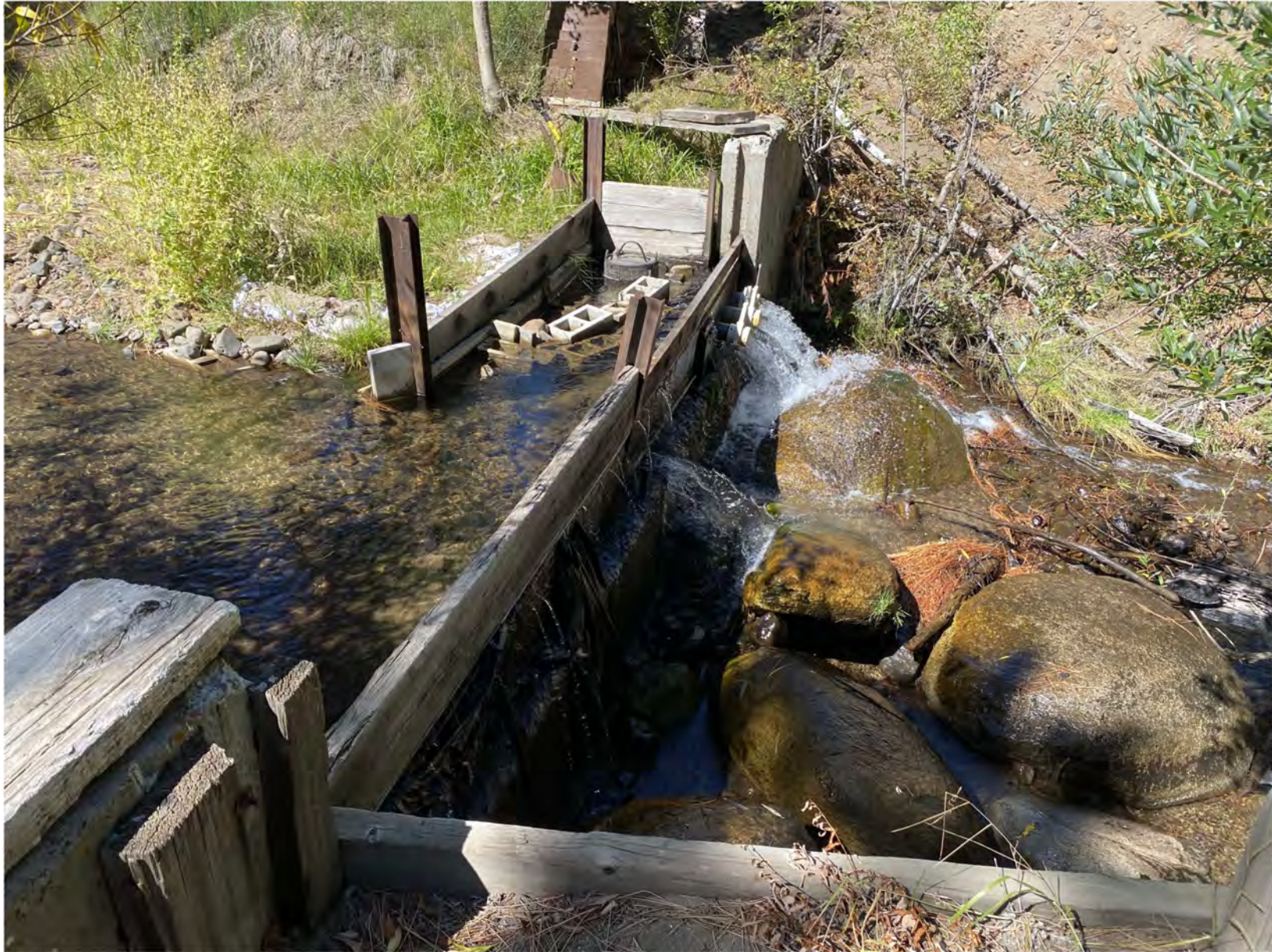
Photo 3: Image of MWC's intake structure from September 26, 2024, depicting modifications that have been made to the intake dam following the 2021 Tamarack Fire.
